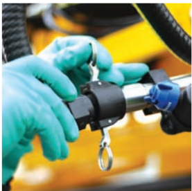
Spray line quick release drain point
